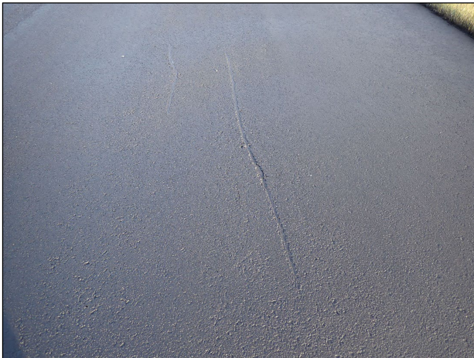
TW-02-04: L&T Cracking
