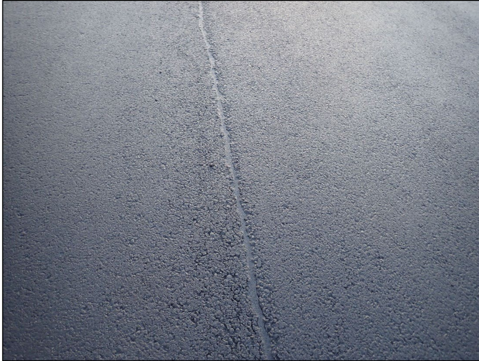
RW05-12-03: L&T Cracking
